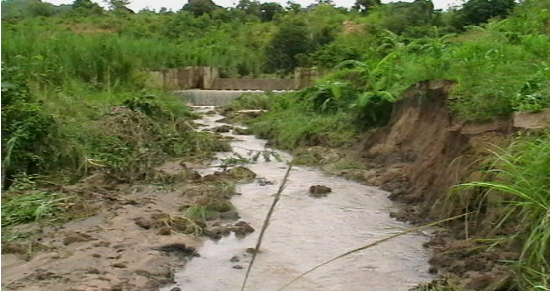
Plate 2: A main canal in KIMBANDE irrigation scheme destroyed by high rainfall
